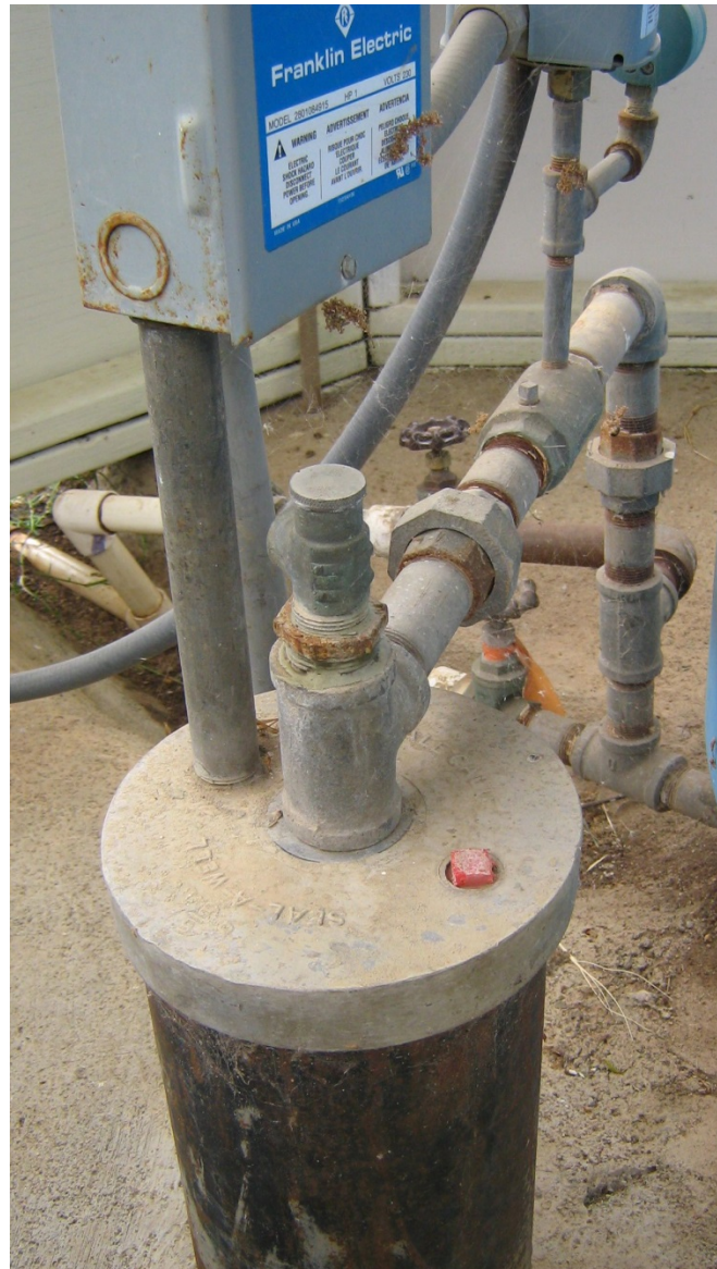
Figure 9. Photo: A domestic well showing the well casing, cover, and conveyance system.
